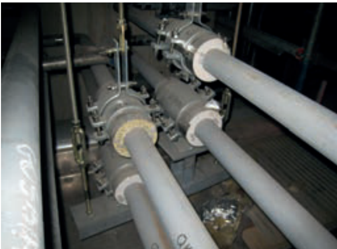
Pipes held in position with cryogenic supports
