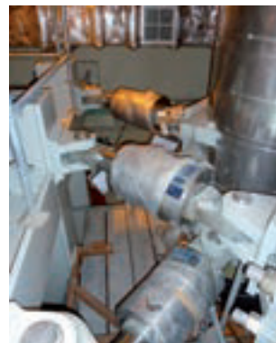
Securing pipe systems with snubbers type 30
