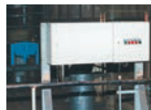
Servohanger switch cabinet
