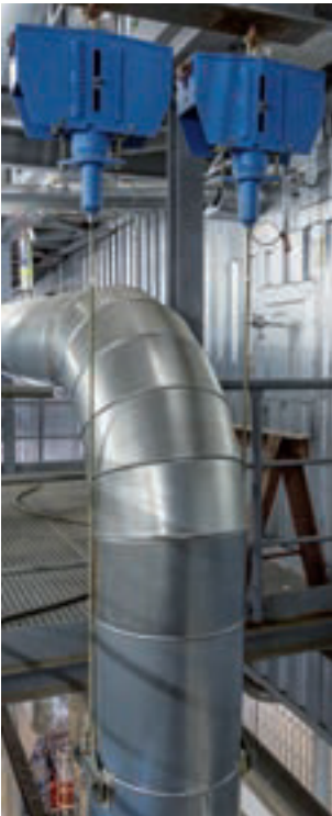
Constant hanger in a coal-fired power station
