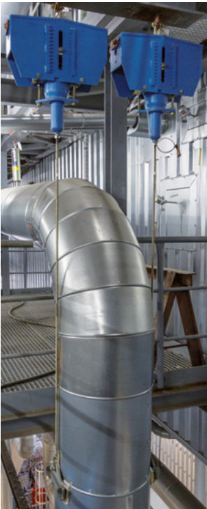
Constant hanger in a coal-fired power station
