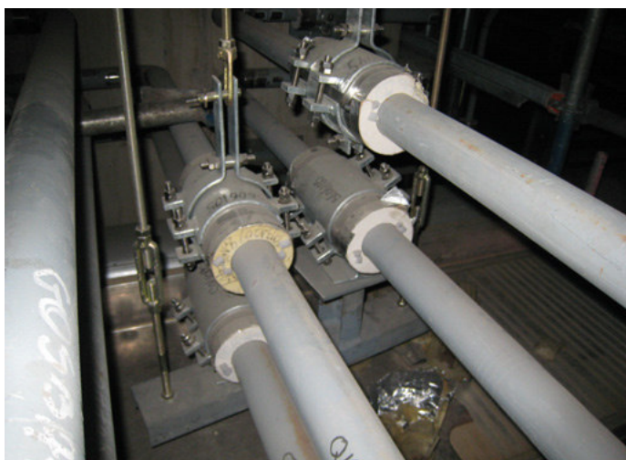
Pipes held in position with cryogenic supports
