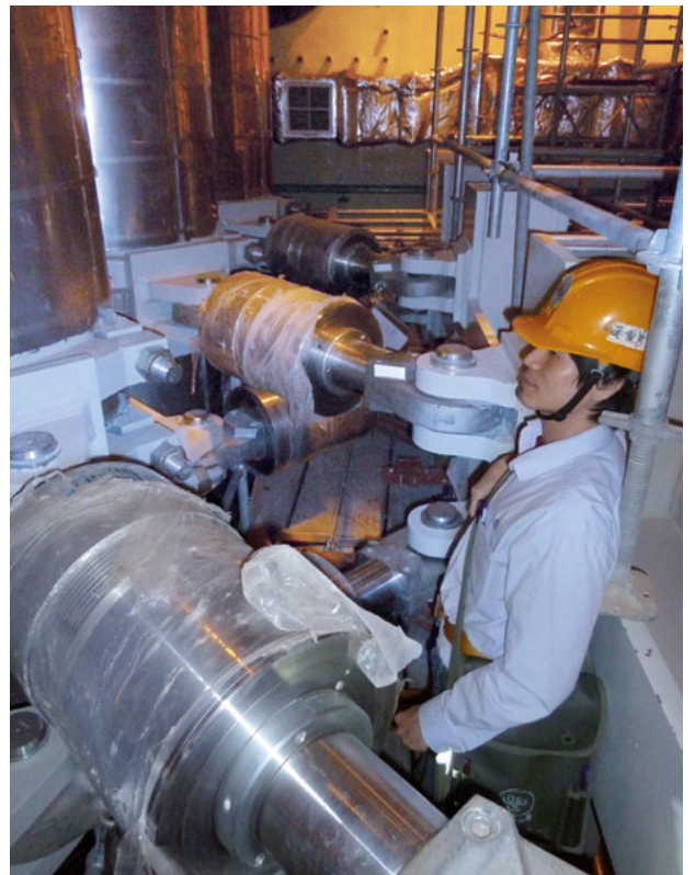
Commissioning of type 30
