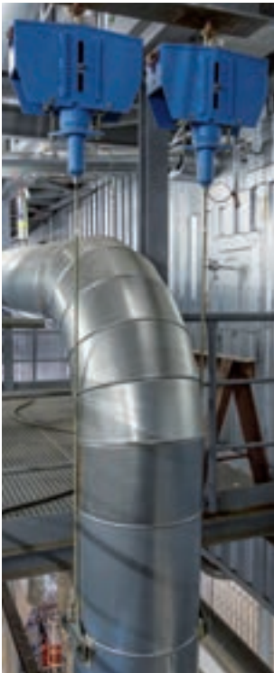
Constant hanger in a coal-fired power station
