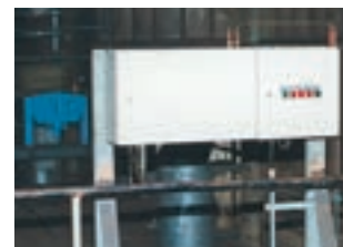
Servohanger switch cabinet
