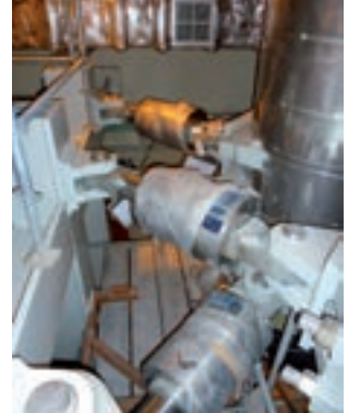
Securing pipe systems with snubbers type 30
