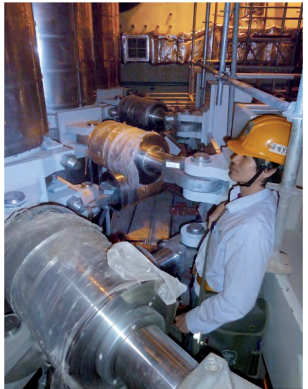
Commissioning of type 30
