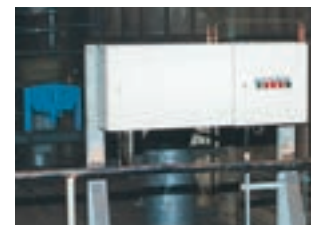
Servohanger switch cabinet
