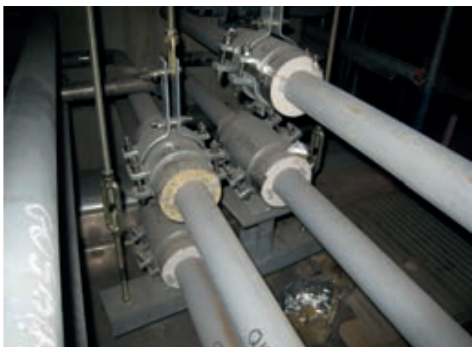
Pipes held in position with cryogenic supports
