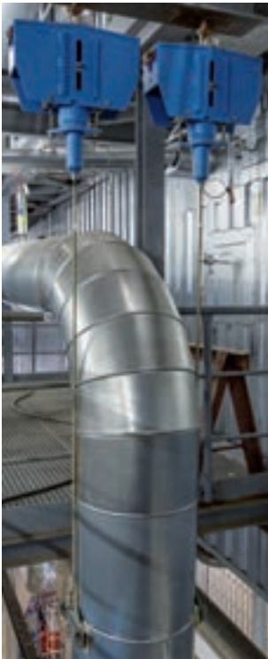
Constant hanger in a coal-fired power station
