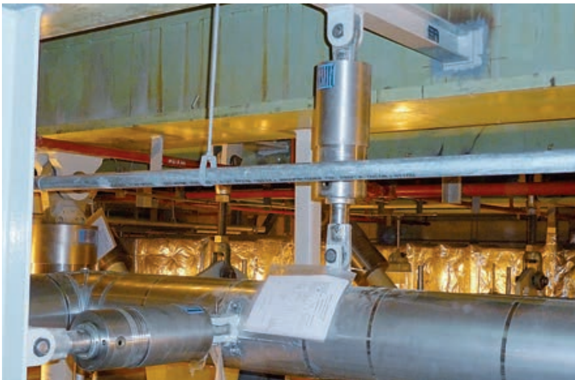
Pipe system secured with snubber type 30 on dynamic clamps type 36
