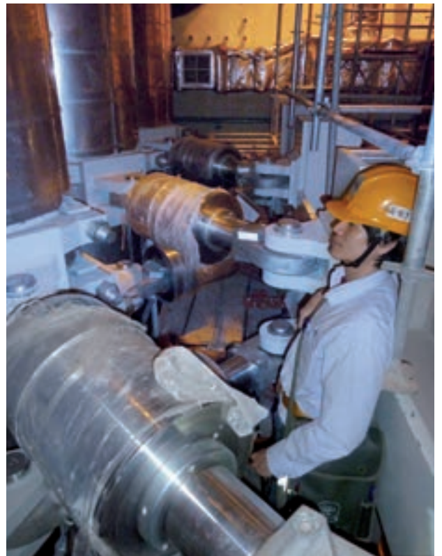
Commissioning of type 30
