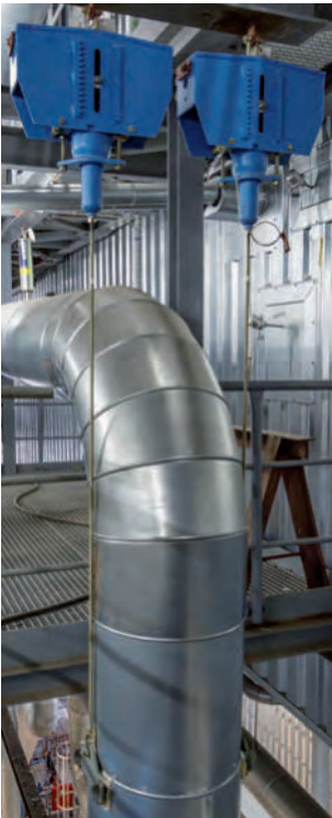
Constant hanger in a coal-fired power station
