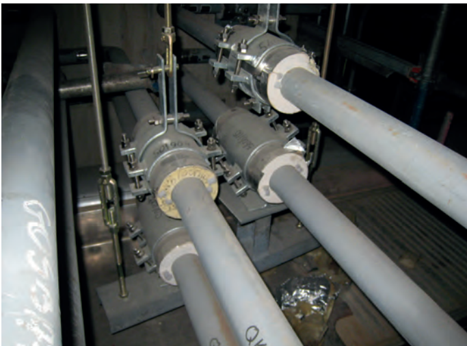
Pipes held in position with cryogenic supports
