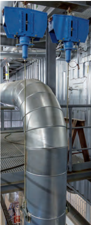
Constant hanger in a coal-fired power station
