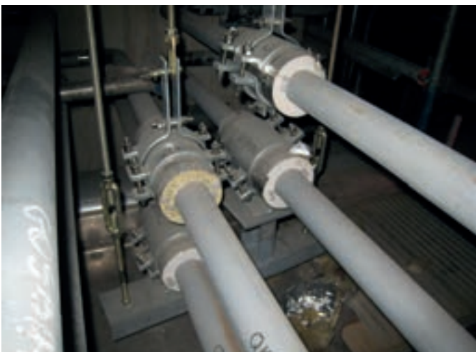
Pipes held in position with cryogenic supports
