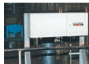
Servohanger switch cabinet
