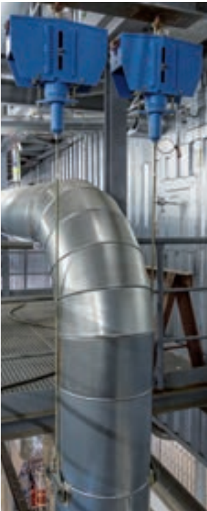
Constant hanger in a coal-fired power station
