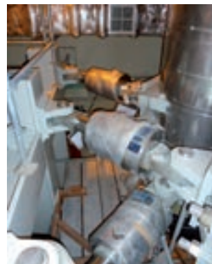
Securing pipe systems with snubbers type 30
